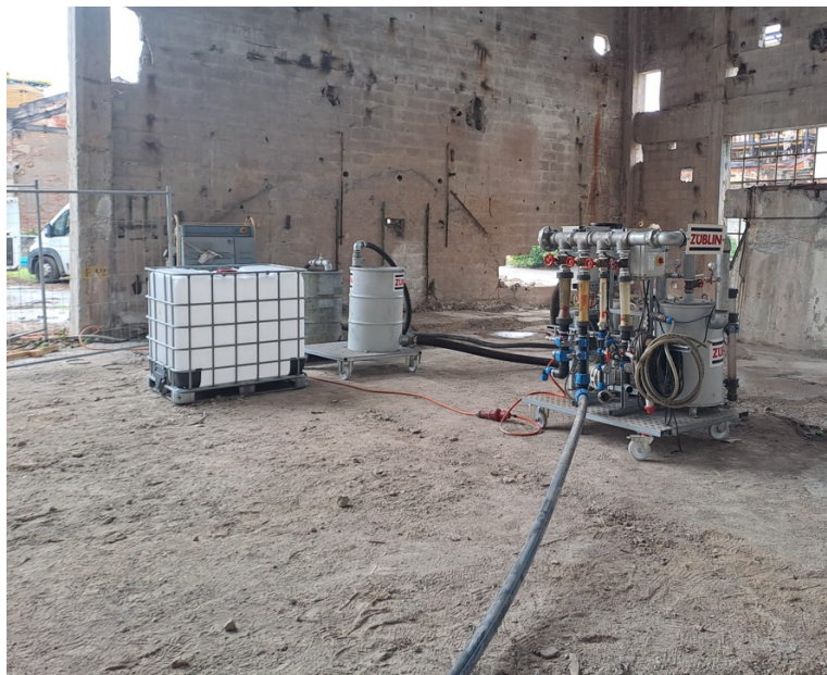
Figura 3: Impianto Soil Vapor Extraction (SVE)
