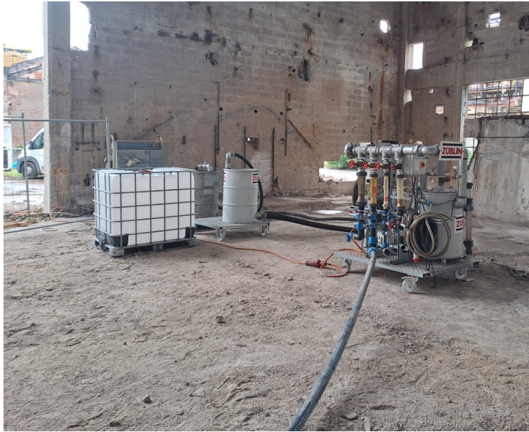
Figura 3: Impianto Soil Vapor Extraction (SVE)
