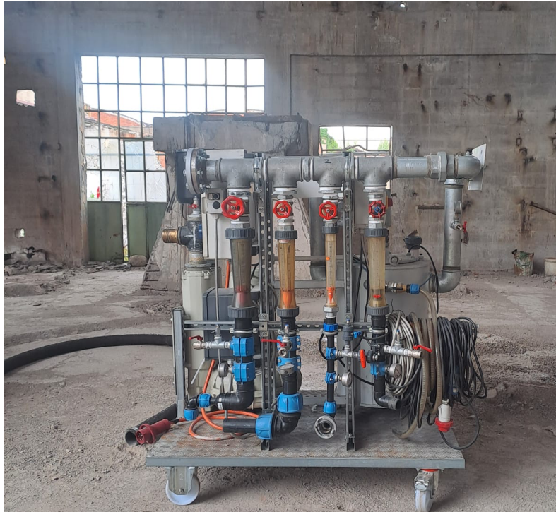
Figura 2: Impianto Soil Vapor Extraction (SVE)
